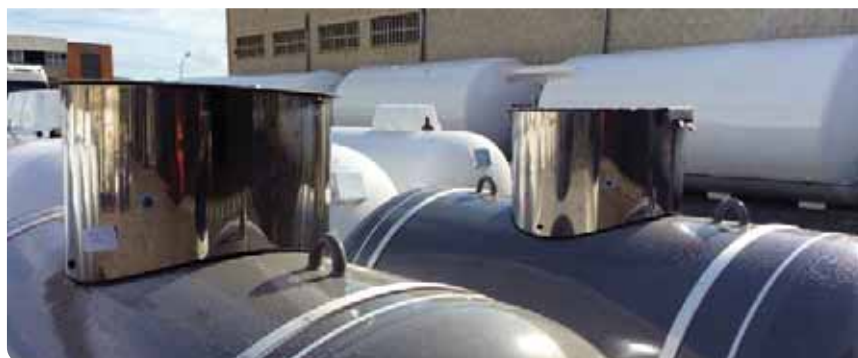
INSPECTION CHAMBERS ON UNDERGROUND TANKS
